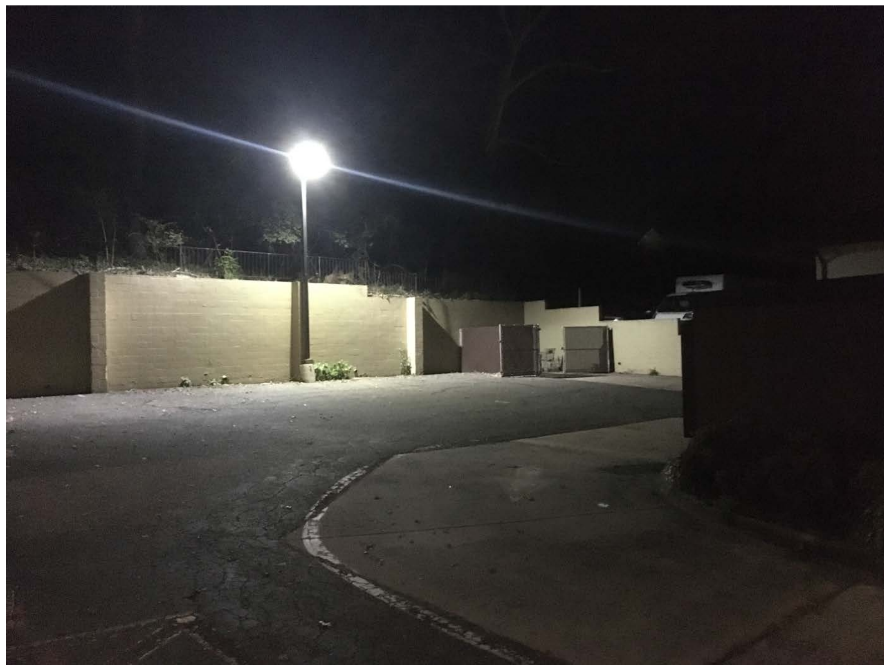
EXISTING REAR POLE LIGHT
