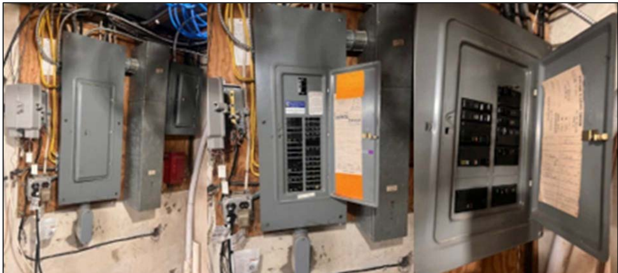
Freeman Store Electrical Panel
