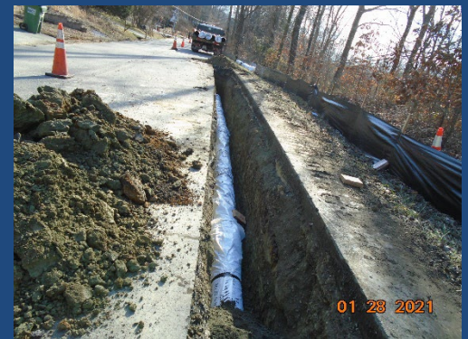
Possum Point Water Main, PWCSA
