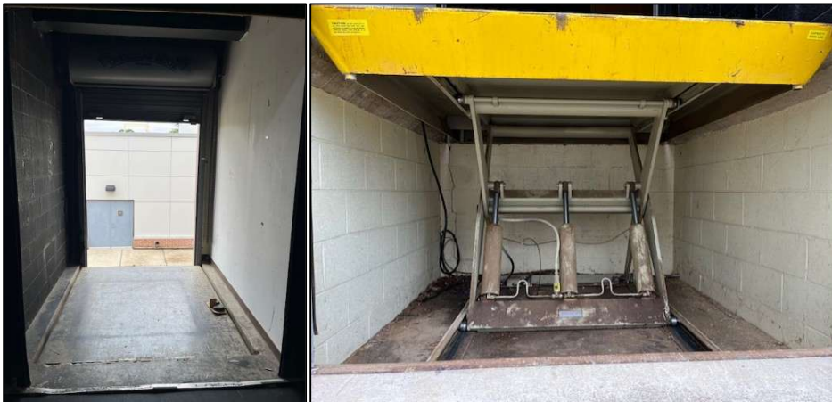
Auditorium Hydraulic Loading Dock
