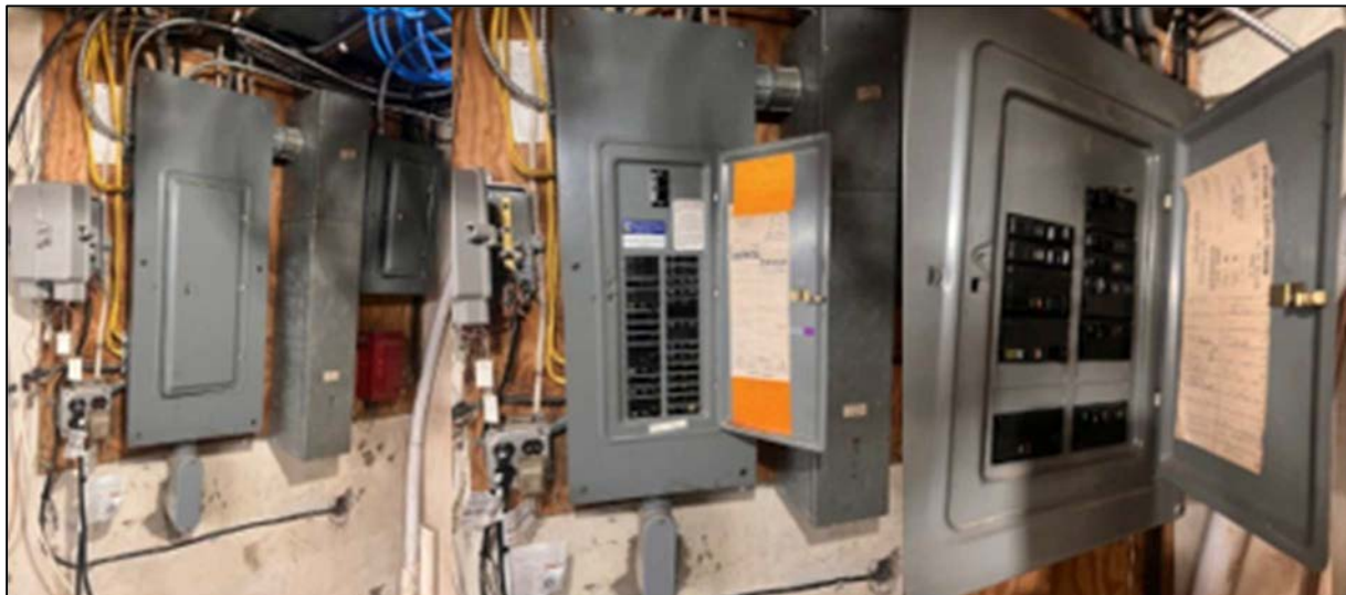
Freeman Store Electrical Panel
