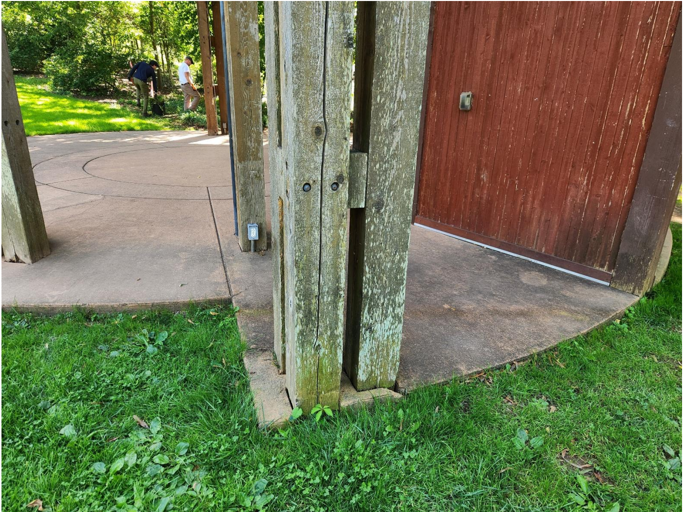
Figure 3 – Existing triple-column set with section loss at base and splitting along column length
