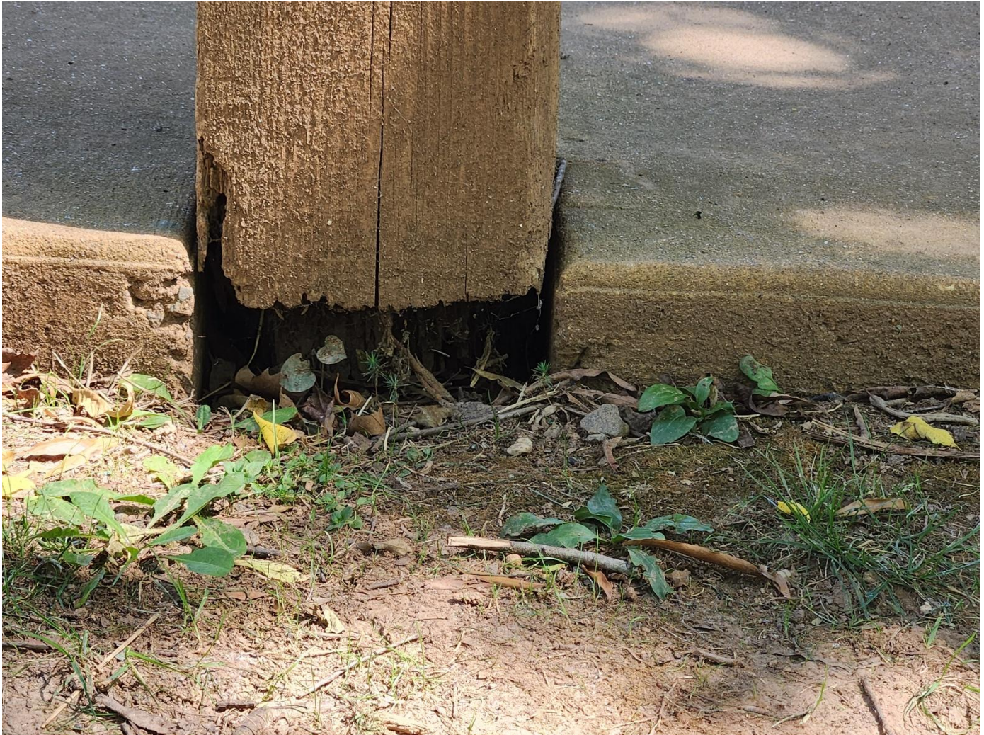
Figure 4 – Close view of section loss at base of wood column
