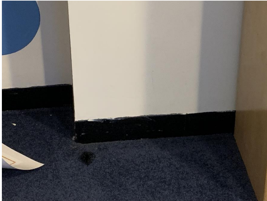
Homogeneous Material No. 12 – Non-ACM 4" Black Vinyl Cove Base with associated tan mastic located in Room 3 adjoining Sanctuary on the upper level.
