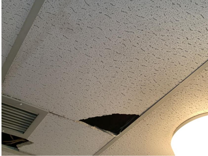
Homogeneous Material No. 9 – Non-ACM White 2' by 4' Lay-in Ceiling Tile with Fissures Design located in Rooms 1 and 2 adjoining Sanctuary.
