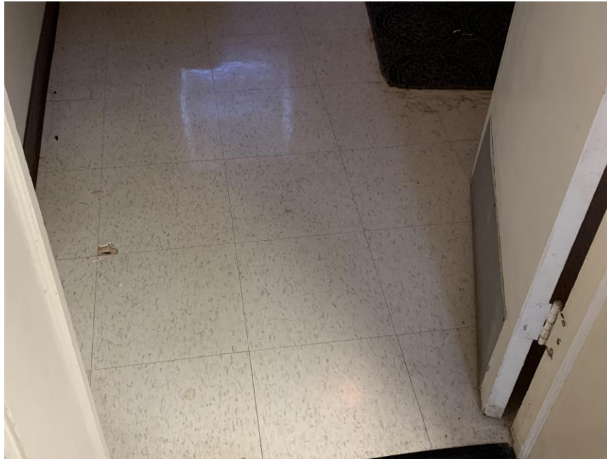
Homogeneous Material No. 20 – Non-ACM Cream mottled 12" by 12" Vinyl Floor Tile with associated cream mastic located in Girl's restroom near the rear foyer area (original building construction).
