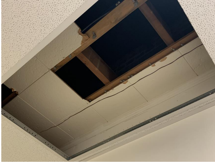
Homogeneous Material No. 19 – Non-ACM White 1' by 1' Lay-in- Ceiling Tile located throughout 1 st floor corridor near the rear foyer area (original building construction).
