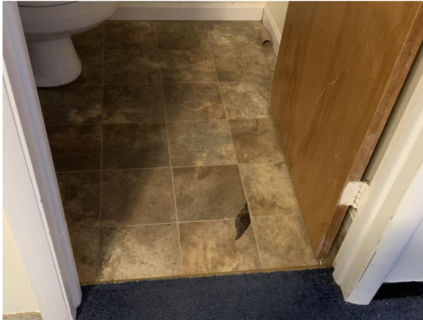
Homogeneous Material No. 14 – Non-ACM Brown square pattern Resilient Sheet Flooring located in Restroom adjacent to the sanctuary and the rear Foyer of the building.
