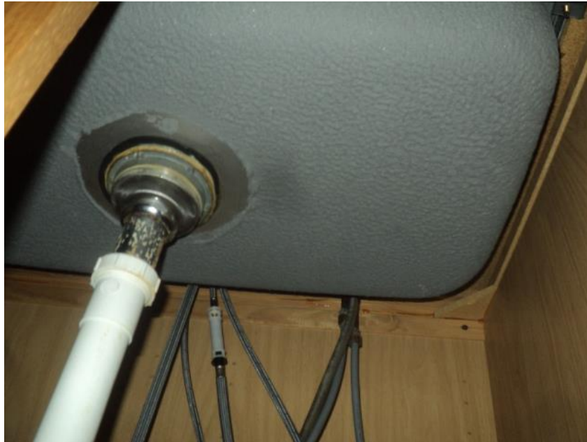
Homogeneous Material No. 24 – Non-ACM Gray Sink Bowl Mastic Coating located in the Kitchen area adjacent to multi-Purpose Room.
