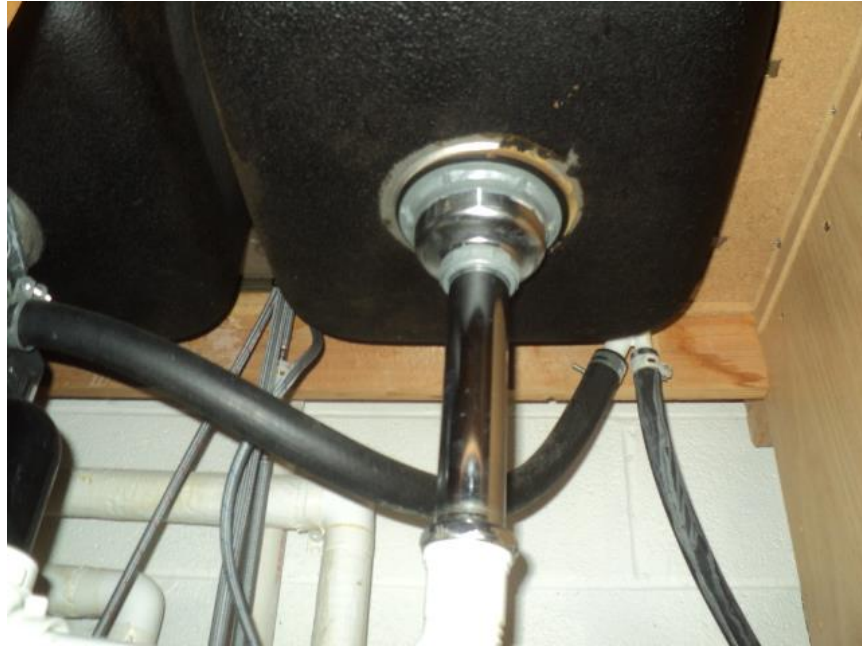
Homogeneous Material No. 25 – ACM Black Sink Bowl Mastic Coating located in the Kitchen area adjacent to multi-Purpose Room.
