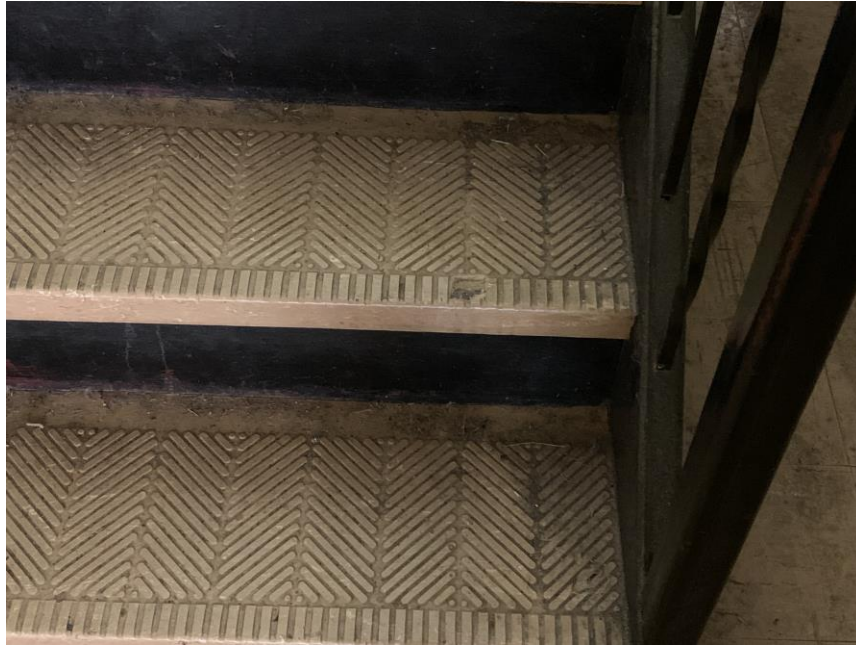
Homogeneous Material No. 17 – Non-ACM Tan Vinyl Stair Tread with associated Tan Mastic located in Stairwell leading to 2 nd floor near rear foyer area (original building construction).
