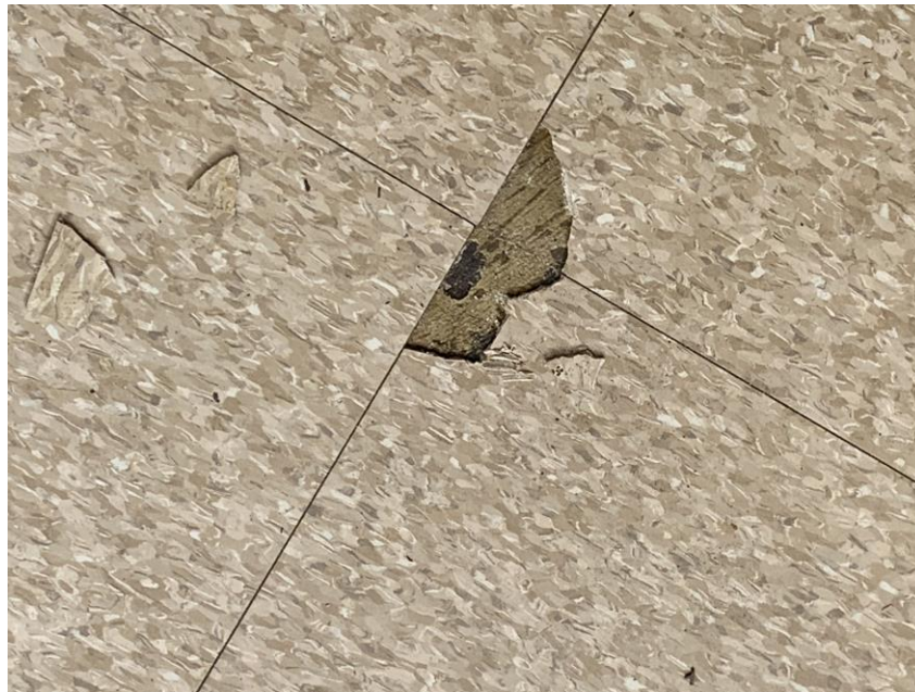
Homogeneous Material No. 28 – Non-ACM Brown mottled 12" by 12" Vinyl Floor Tile with associated tan/black Mastic located in 2 nd Floor Classroom 1 (original building construction).
