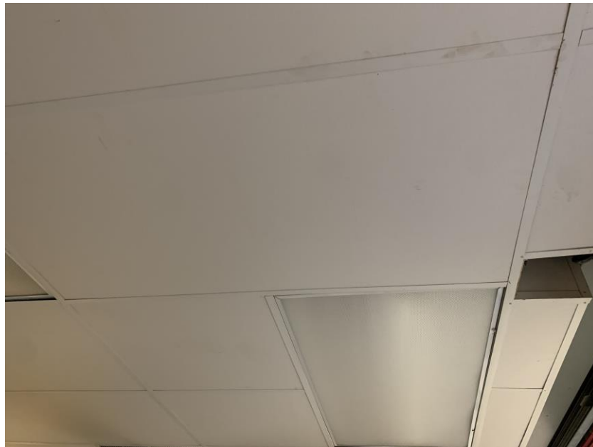
Homogeneous Material No. 26 – Non-ACM White Gypsum 2' by 4' Ceiling Tile located in the Kitchen area adjacent to multi-Purpose Room.
