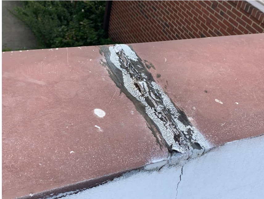
Homogeneous Material No. 3 – Non-ACM Black/Gray Parapet Wall Cap Caulk located on Shingle Roof over the Sanctuary.
