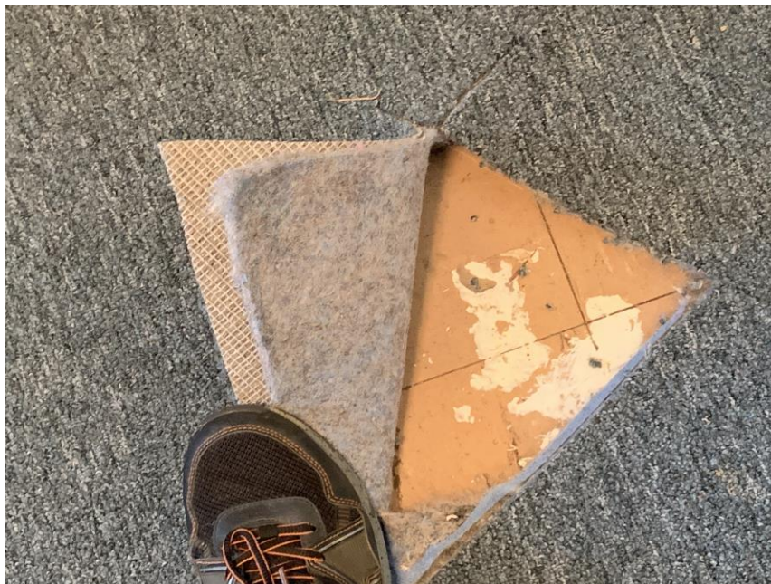
Homogeneous Material No. 7 – ACM 9" by 9" Tan Vinyl Floor Tile with Associated Black Mastic located under carpeting in Rooms 1 and 2 Adjoining the Sanctuary and on 2 nd floor (original building construction).
