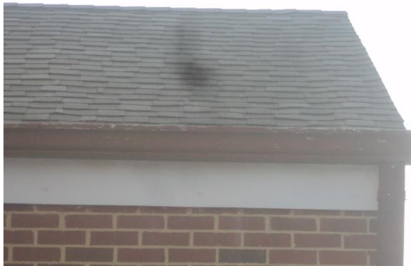
Homogeneous Material No. 5 – Non-ACM Black Asphalt Shingle with Black Felt Paper located on Shingle Roof over Original Building Construction.
