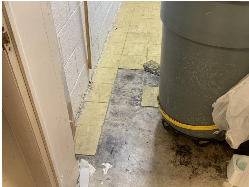
Homogeneous Material No. 18 – ACM Cream 9" by 9" Vinyl floor Tile with associated black mastic located in the 1 st floor storage room across from the rear foyer area.
