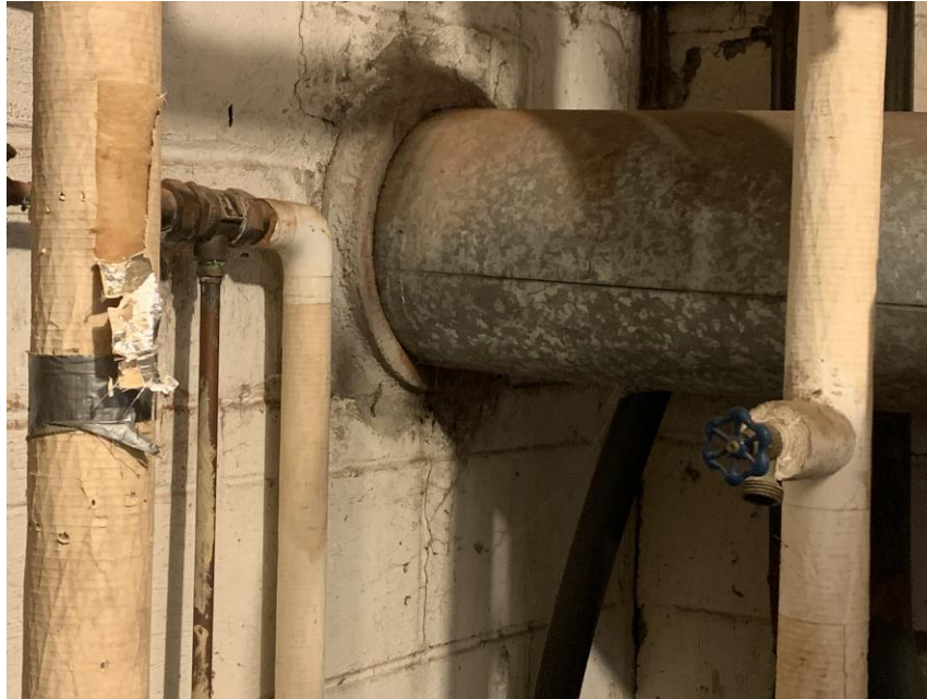
Homogeneous Material No. 23 – Non-ACM Gray Boiler Flue Pipe Wall Packing located in the Mechanical Room.
