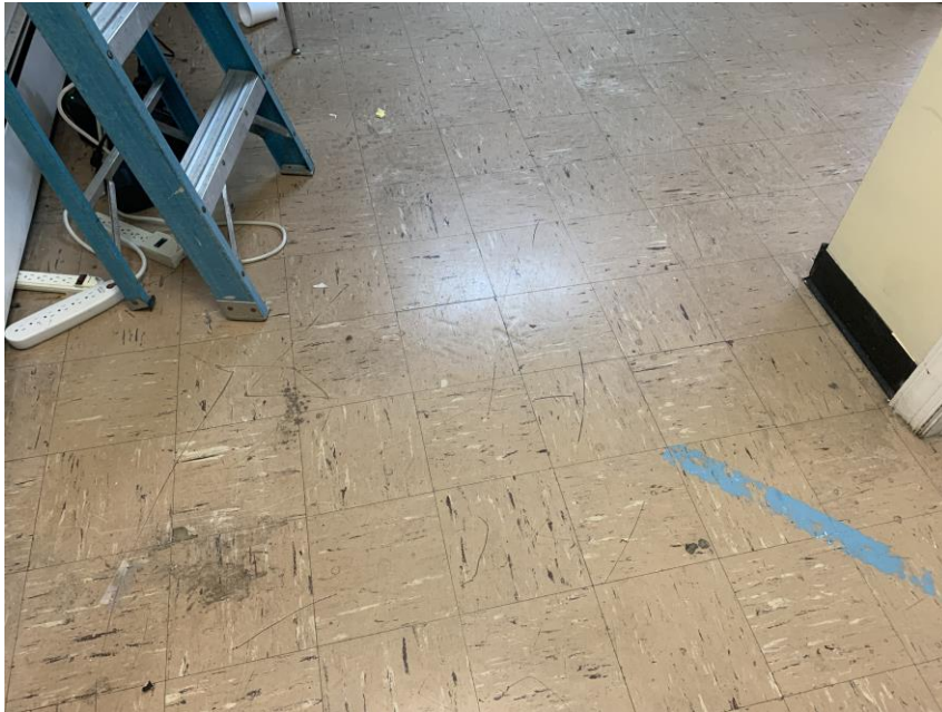
Homogeneous Material No. 30 – ACM Tan with brown streaks 9" by 9" Vinyl Floor Tile with associated black mastic located in the 2 nd Floor Corridor, classrooms and throughout the original building construction.
