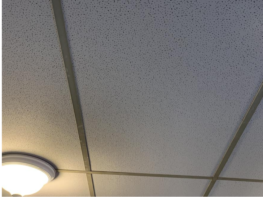
Homogeneous Material No. 13 – Non-ACM White 2' by 4' Lay-in Ceiling Tile with Pin Dots Design located in Room 3 adjoining Sanctuary on the upper level.
