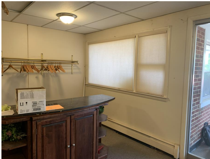
Homogeneous Material No. 16 – ACM White Drywall with Associated White Joint Compound, White Tape and White Paint located in the Girls' and Boys' restroom near Rear Foyer area of the building and throughout the original building construction on 1 st and 2 nd floor.
