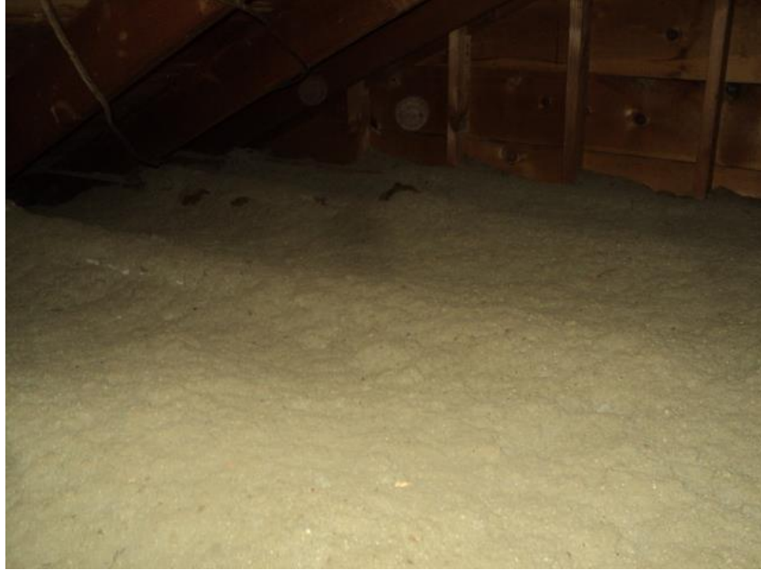
Homogeneous Material No. 29 – Non-ACM Tan Blown-in Attic Insulation located in the Attic on the 2 nd floor (original building construction)..
