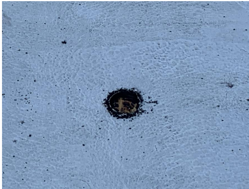
Homogeneous Material No. 6 – Non-ACM Built-up Black Asphalt Roof Field located on Portico flat roof at rear of the building.
