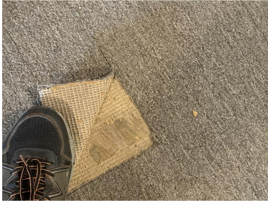
Homogeneous Material No. 15 – Non-ACM Tan Carpet Glue located in the rear Foyer of the building.
