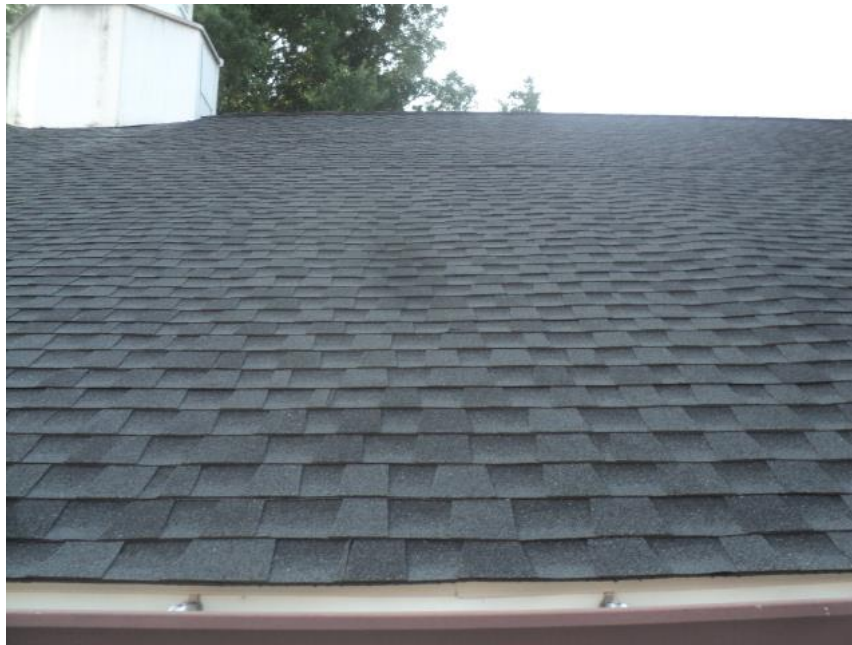
Homogeneous Material No. 4 – Non-ACM Black Asphalt Shingle with Black Felt Paper located on Shingle Roof over the Sanctuary.
