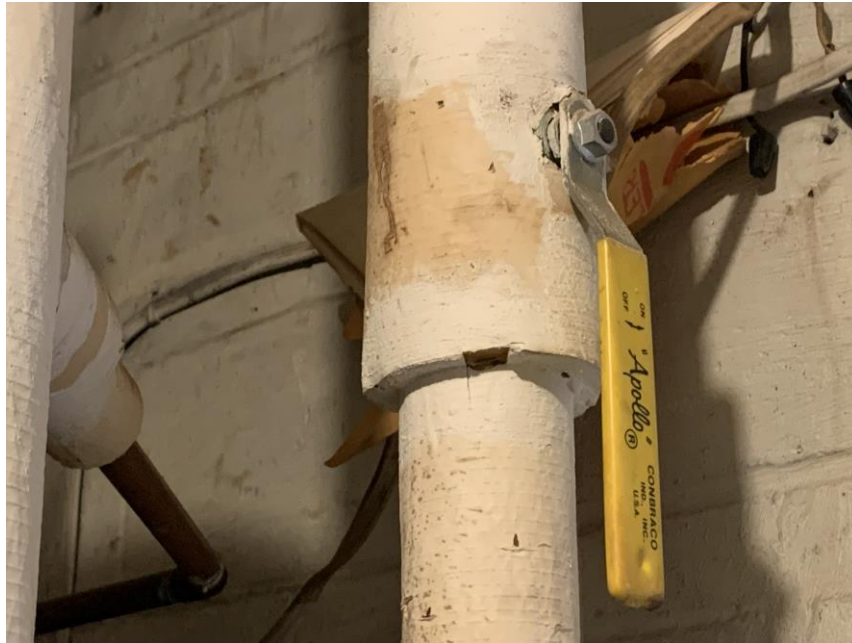
Homogeneous Material No. 22 – Non-ACM White Pipe insulation Mastic located in the Mechanical Room.
