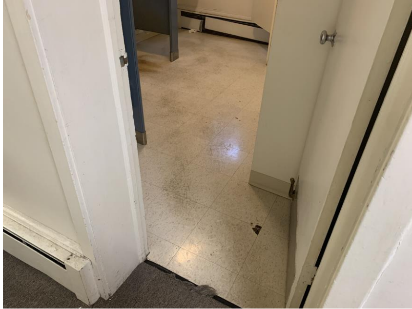
Homogeneous Material No. 21 – Non-ACM Cream mottled 12” by 12” Vinyl Floor Tile with associated Black mastic located in Boy’s restroom near the rear foyer area (original building construction).
