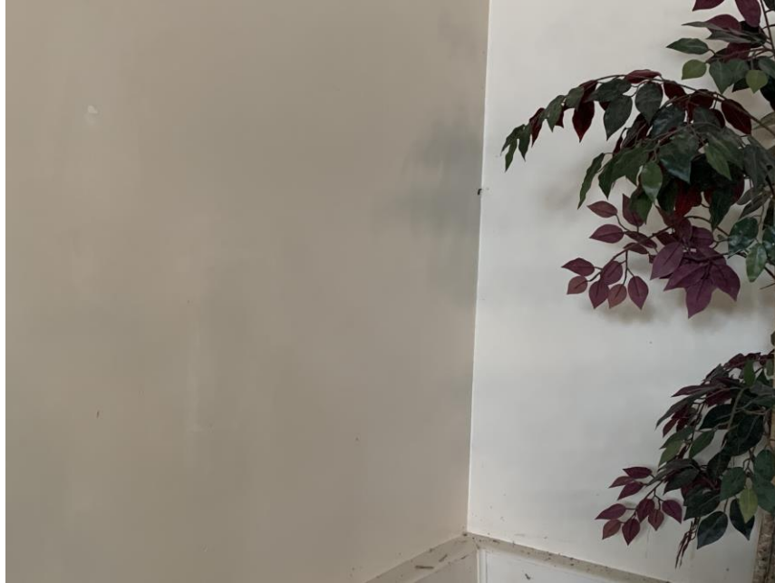
Homogeneous Material No. 11 – Non-ACM White Drywall with Associated White Joint Compound and White Paint located Throughout Sanctuary and Adjoining Rooms.
