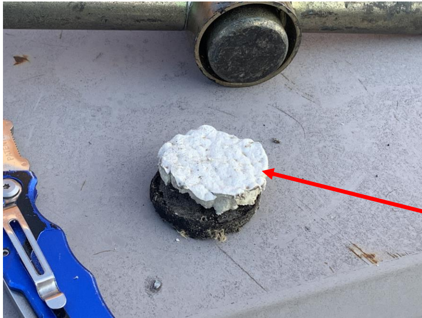
Homogeneous Material No. 1 – Non-ACM Built-up Roof Field with yellow insulation located on the building roof (flat part).
