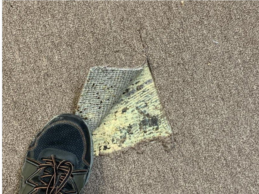
Homogeneous Material No. 27 – Non-ACM Yellow Carpet Glue mixed in with Black Mastic located in Classroom 2 adjacent to multi-purpose Room.
