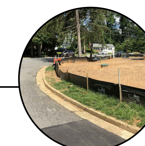
This photo shows the "bend" in the mainstem portion of the street. The developer of #914 has cleared the frontage; however, he plans to add landscaping and tree(s) later in construction.
